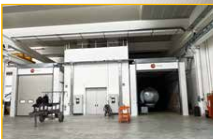
REPARTO VERNICIATURA VARNISHING DIVISION
